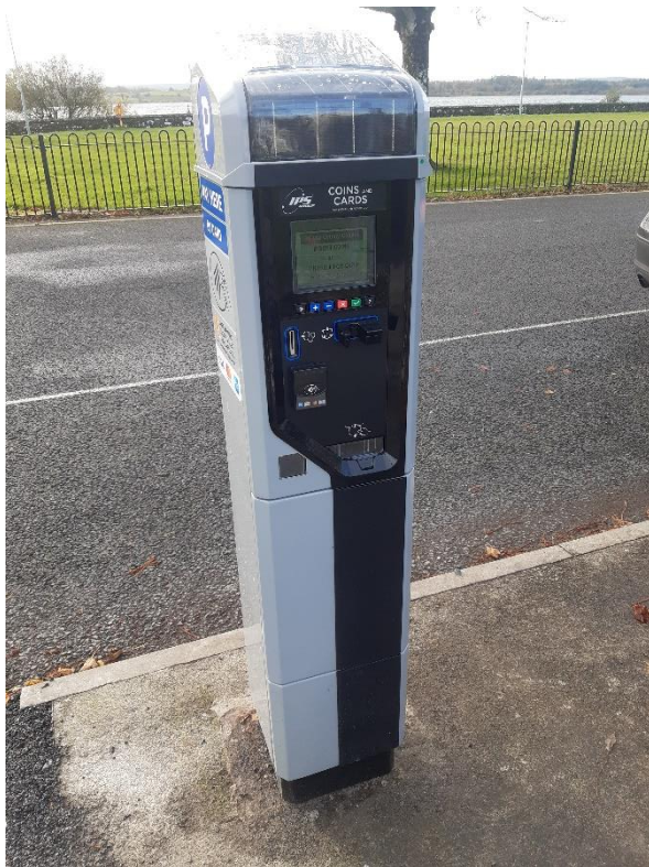
New Unit Installed in Loughrea
