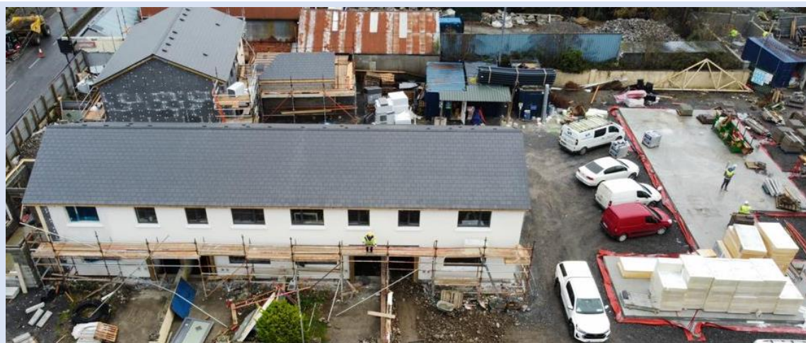
Bridge Court, Ahascragh. Redevelopment and new Build, LA Build programme. Completion Mid 2023.
